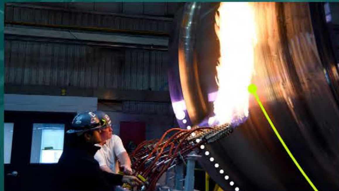
Fabrication work is underway on the reactor pressure vessel for the first SMR at the Clarington, Ontario site.
