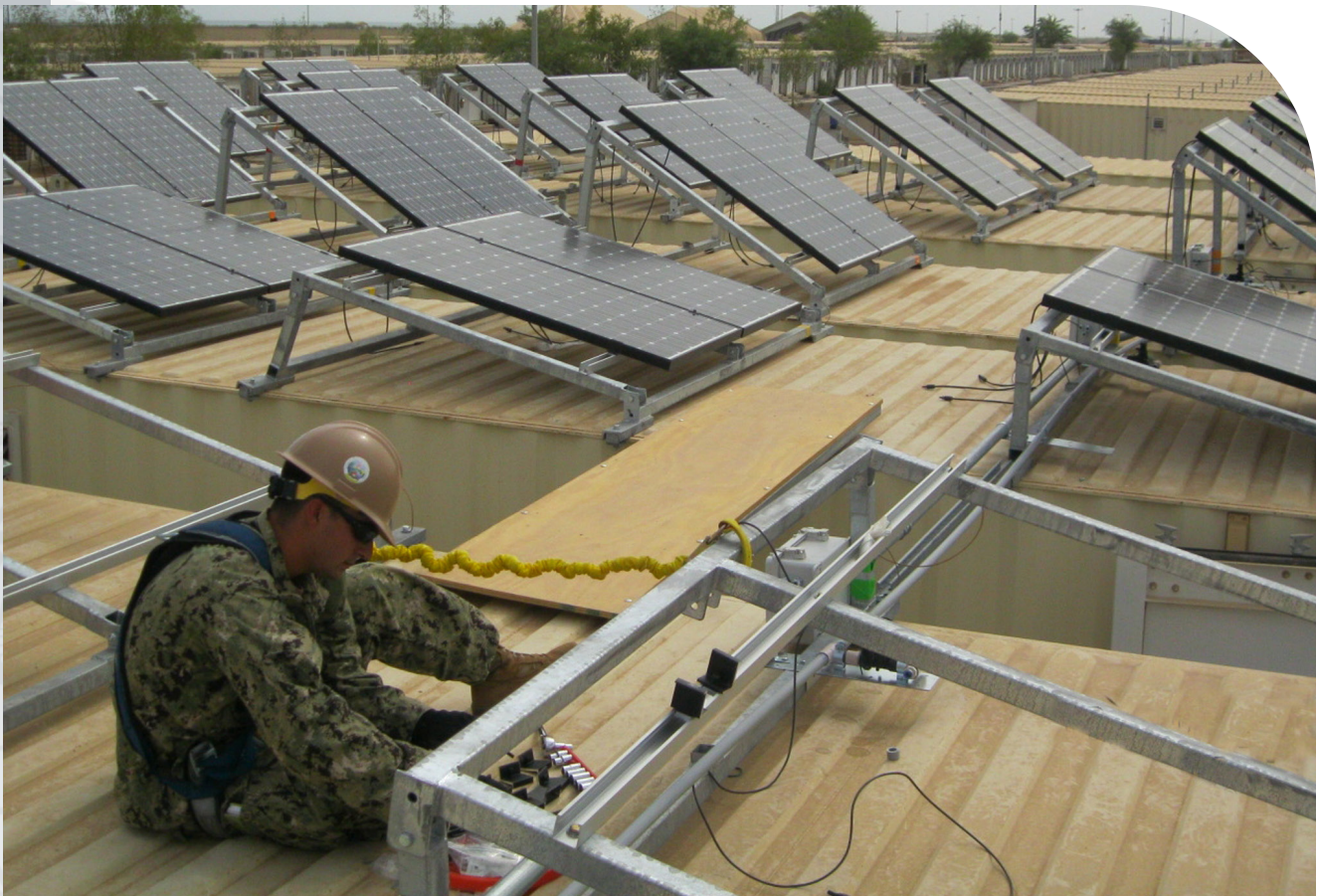
A Sailor with Naval Mobile Construction Battalion 1 (NMCB1) installs a water wash valve atop a containerized living unit at Camp Lemonnier in Djibouti, Africa. NMCB1 installed the arrays to study how the impacts of wind and dust affect the arrays' effectiveness. Solar arrays reduce the base's electrical load and the amount of diesel fuel used to power generators, Sept. 12, 2012.
