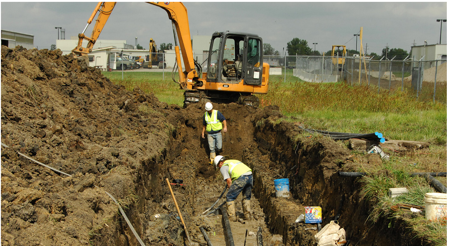
Workers prepare to splice a “T” pipe while installing a geothermal system at Selfridge Air National Guard Base, Michigan, September 29, 2011. (Department of Air Force photo by John Swanson)
