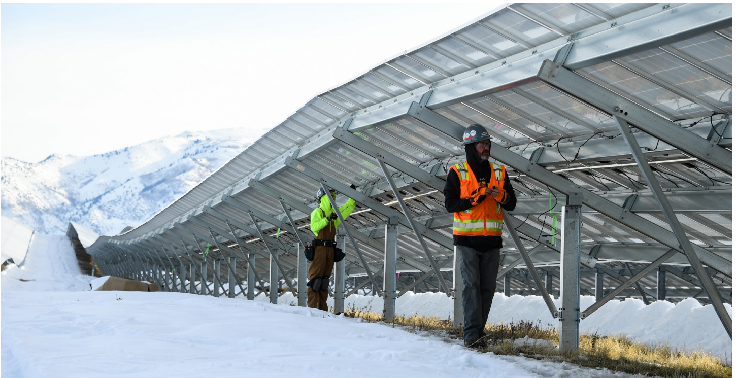
The solar array installed at Hill Air Force Base, Utah, in 2018 increased the amount of renewable energy produced on base and will be incorporated into future microgrid planning. The new system was installed through an Energy Savings Performance Contract that costs the government no upfront money. Energy Solutions Group will operate and maintain the system during the 23-year arrangement. Pictures show a conduit line being installed and electrical wiring clips attached to the new panels. (Department of Air Force photo by R. Nial Bradshaw)
