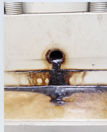
Open port on Fuel Control Valve Actuator
