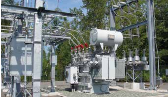
Lex Engineering design for a BC Hydro 69 kV, 25 MVA substation at Langley, British Columbia. Photo courtesy of Lex Engineering.
