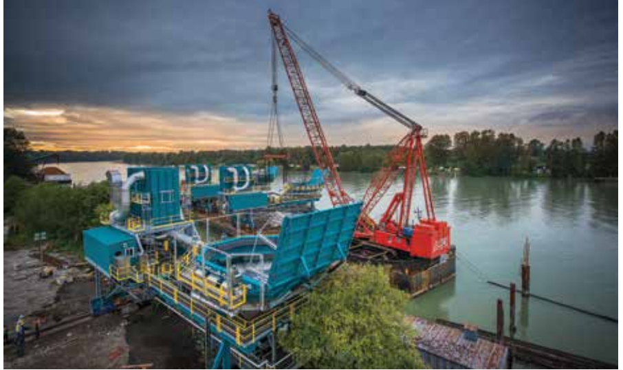
Mobile hoppers being lifted onto Amix’s ArcticTuk barge. Photo courtesy of Amix Heavy Lift.
